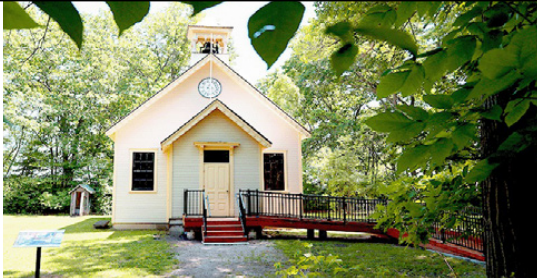
New entry ramps are installed at the Rokeby School (pictured), Cameron Church and Tudhop Cabin to improve accessibility at LHM.
