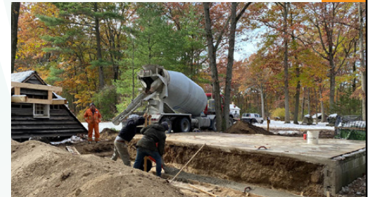
Concrete footings are poured as part of the foundation for the reconstruction of the historic Canatara Cabin at LHM.
