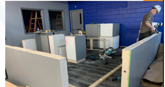
A new accessible service desk is installed as part of the renovations to the former community hall at the Clearwater Arena in Sarnia, in preparation for the opening of the new Clearwater Library, scheduled for February of 2024.
