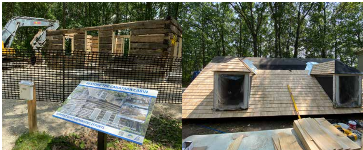
IMAGES: From left - 1) Cabin reconstruction progress in July 2024. 2) Cedar shingles being applied to the cabin roof before it was installed on the main structure, August 2024
