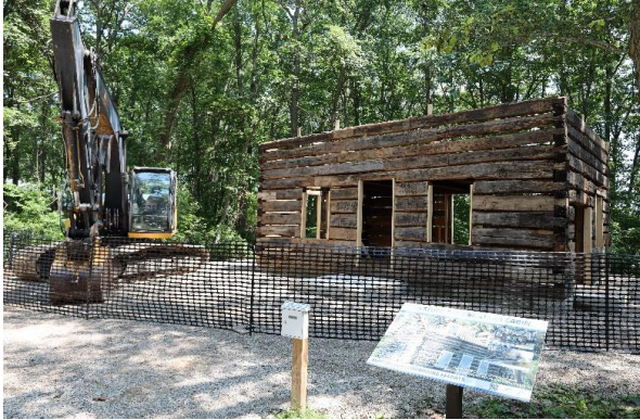
Figure 7 – In June of 2024, work began to reconstruct the cabin log by log on top of the modified foundation.
