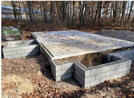
Figure 2 - The concrete block footings of the previous program building foundation are modified to suit the footprint of the cabin and a new concrete slab foundation is poured.
