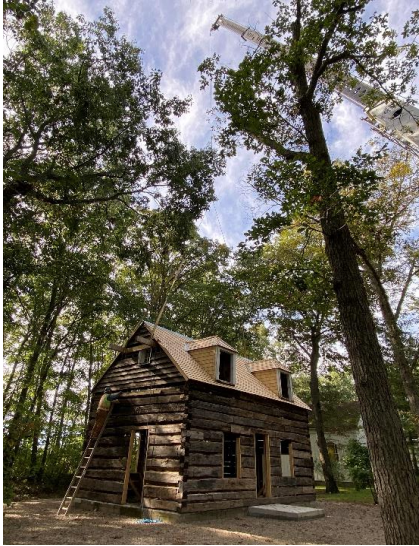
Figure 10 – By the end of September 2024, the structure was beginning to look like a complete cabin when the restored roof was lifted into place and secured to the structure.
