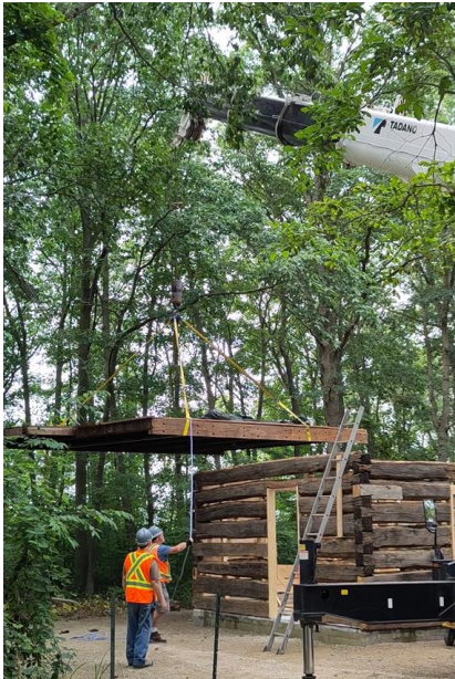
Figure 8 – By July of 2024 the main walls of the structure were complete, and the second floor was hoisted onto the cabin and secured in place to support the remainder of the structure.
