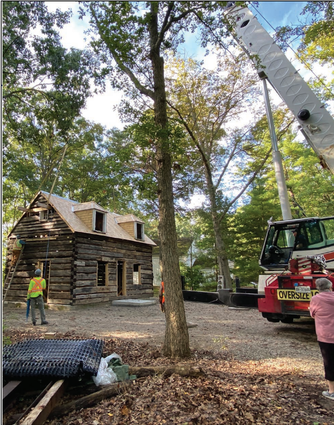
The restored roof is lowered onto Canatara Cabin at Lambton Heritage Museum.
